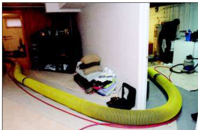
A large hose that provides suction coils through a home in Twin Falls as Camron White, an employee of Air Quality Services, works in the background Thursday.
