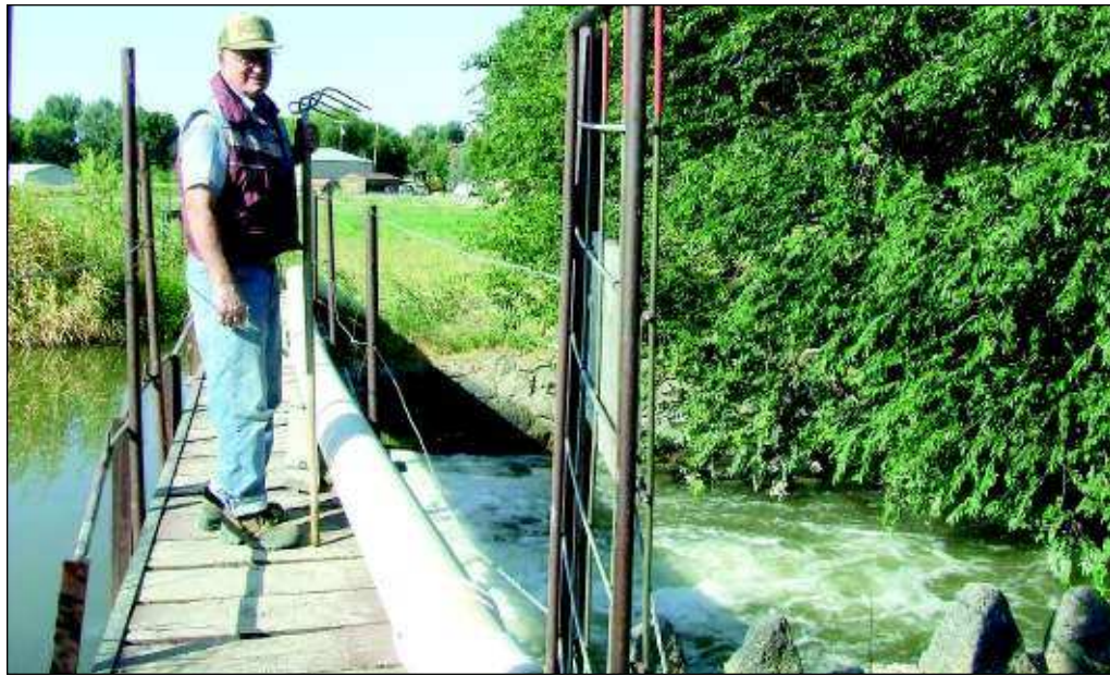
Willie Ruple checks Gooding irrigation gates in the spring of 2008. Gooding officials are holding a series of public meetings to discuss plans to address current and future water needs.
