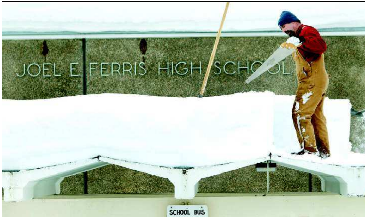
Norm Carveth of the Spokane Public Schools maintenance department uses a handsaw to cut snow into shovel-sized chunks as he helps clear the roof of the bus loading area at Ferris High School in Spokane, Wash. Jan. 5. AP photo
