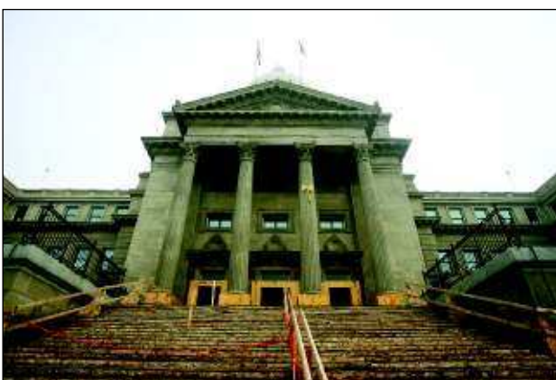
Plywood planks lead to a blocked entrance to the state Capitol building that is under construction.
