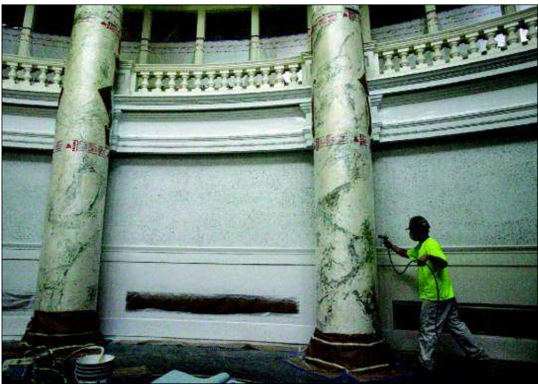
A worker paints the walls between two columns that were painted by immigrants 100 years ago in the Senate chambers room at the state Capitol building in Boise.
