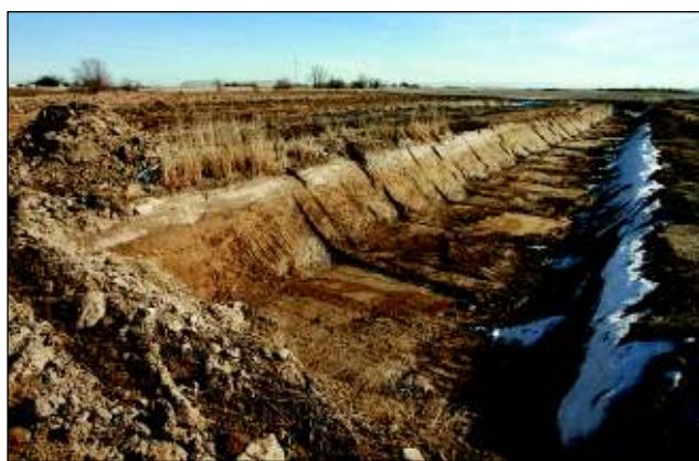
One of 13 settling ponds that will help filter water that runs through the Perrine Coulee.
