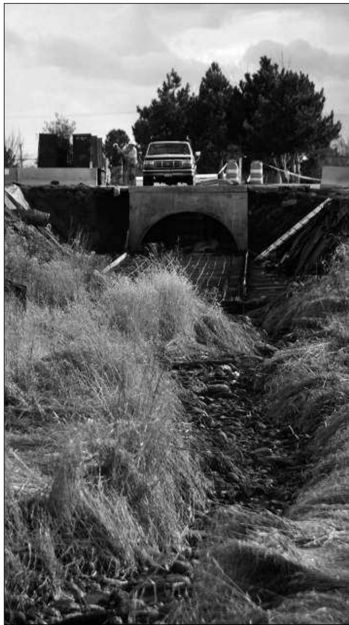
MEAGAN THOMPSON/Times-News Construction workers get to work on a collapsed culvert Wednesday on the west side of Fred Meyer on Fillmore Street in Twin Falls.
