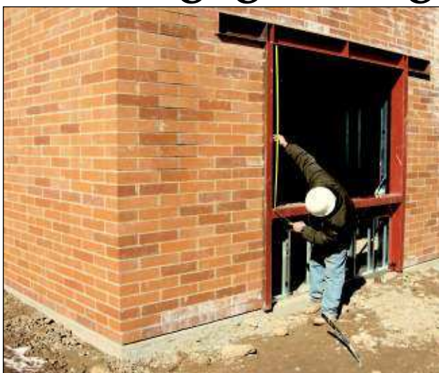
Starr Corp. site Superintendent Larry Pollard works at the construction site of Kimberly Elementary School's new multipurpose building.
