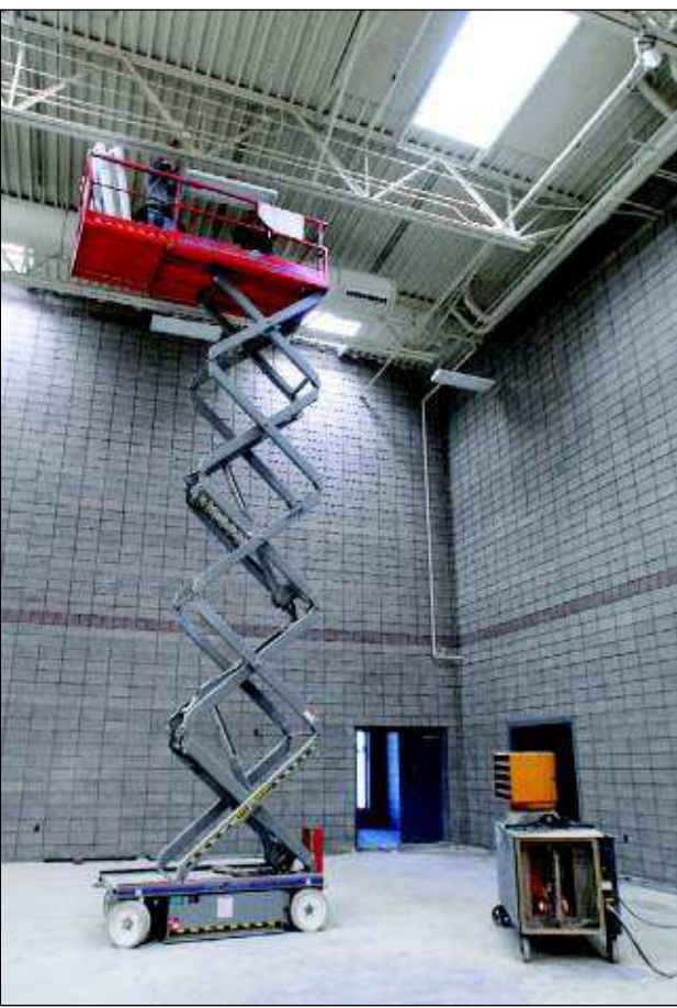
Electricians with Portnuef Electric of Pocatello place a lighting fixture above the secondary basketball court Friday afternoon at Canyon Ridge High School in Twin Falls.
