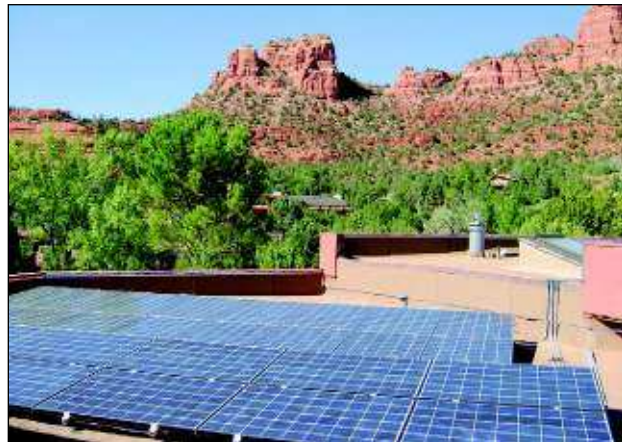
Photo courtesy of Northern AZ Wind & Sun
