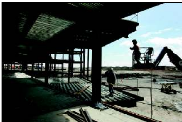
Matt Knighten, right, of Boise Steel Erectors Inc., works on the diagnostic/treatment section of the new hospital Thursday.
