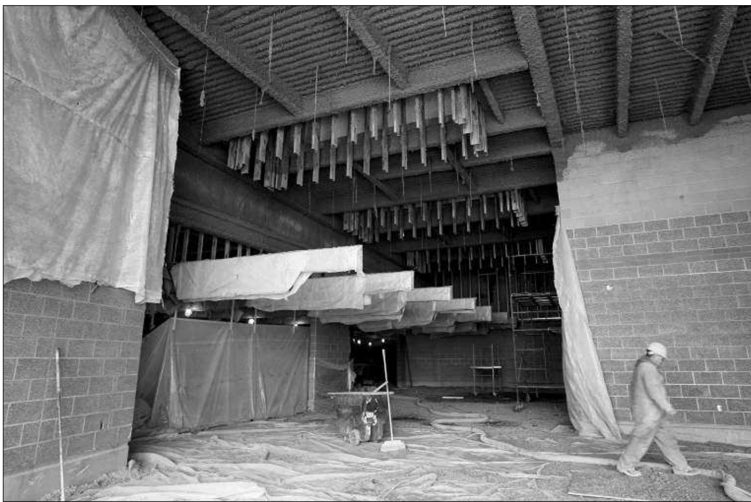
A construction worker walks through the unfinished foyer of Baun Gymnasium at Twin Falls High School.
