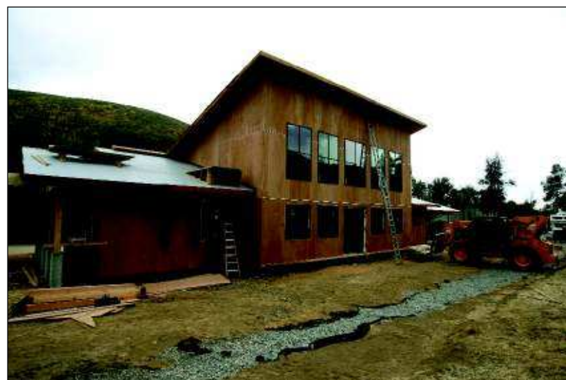
See LODGE, Main 2 A view of the new Soldier Mountain Ski Resort lodge currently under construction.
