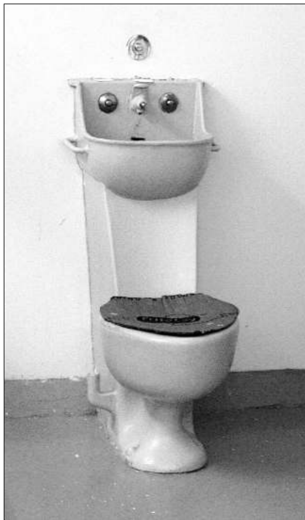
The toilet and sink units at the Jerome County Jail are 30 years old and were received secondhand from the Idaho State Prison in Boise. The cost to replace one unit is up to $5,000 for parts and labor, Sheriff Doug McFall said.
