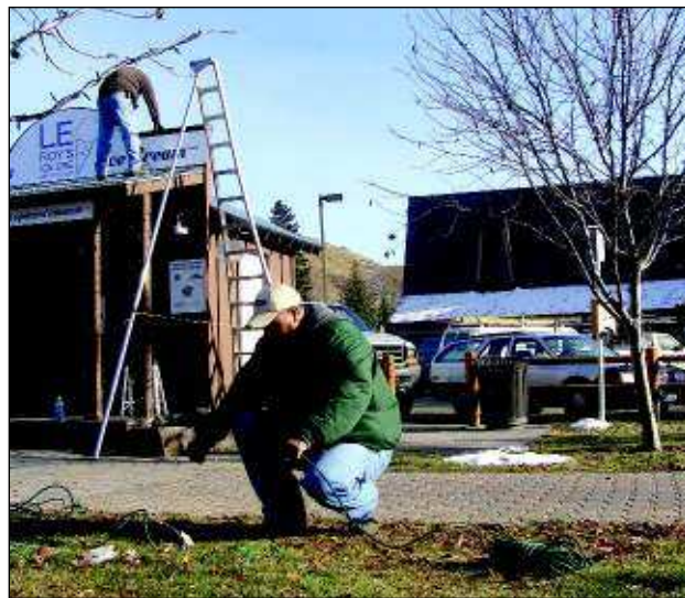
KAREN BOSSICK/For the Times-News Eliceo Patlan prepares to string Christmas lights while Adolfo Rivera works on the roof of LERoy's Ice Cream. The Ketchum ice cream shack occupies property planned to become part of a large town plaza.
