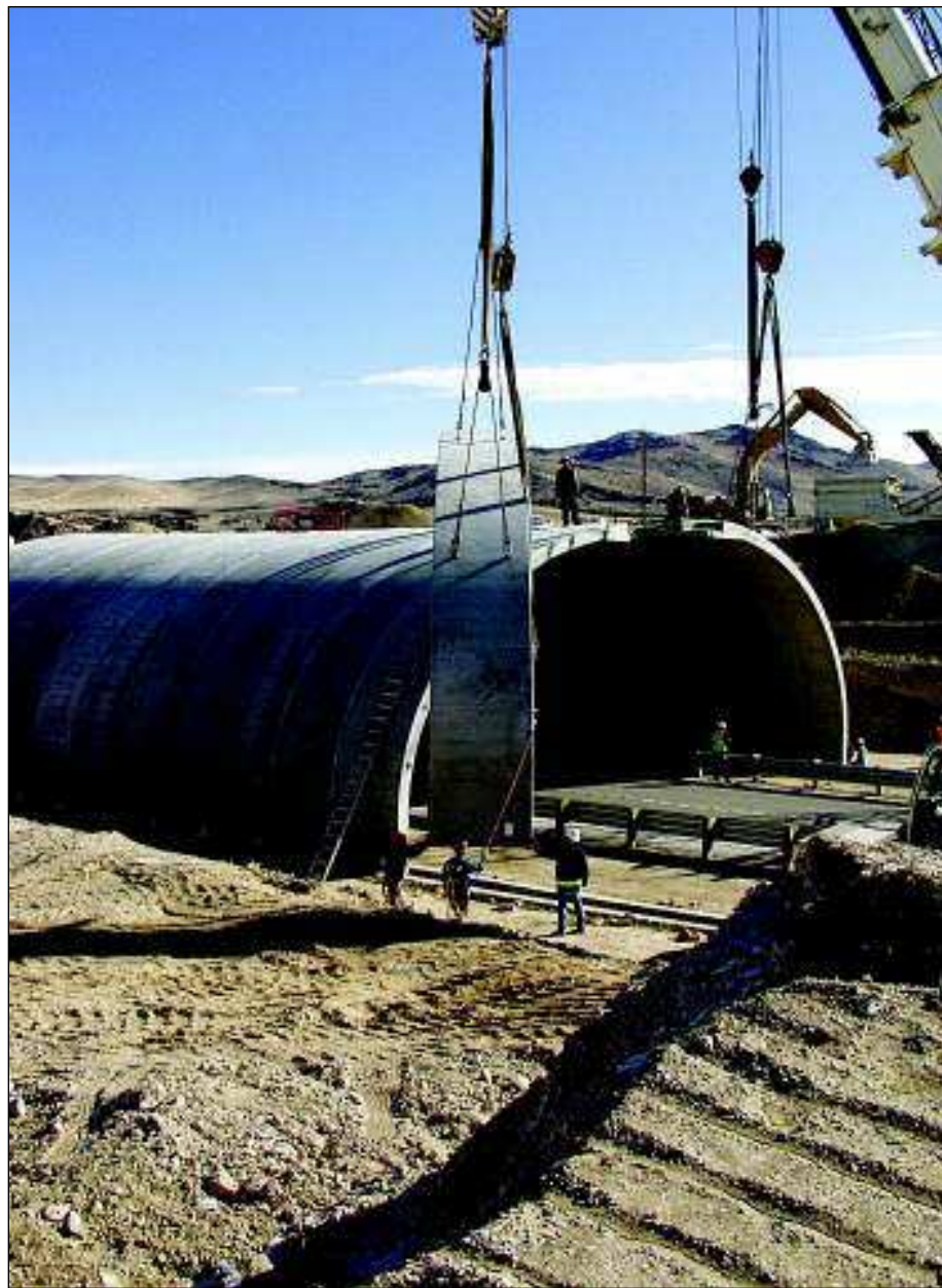
Construction workers hoist half of a prefabricated ring that will serve as part of the wildlife overpass on U.S. Highway 93 about 10 miles north of Wells, Nev.
