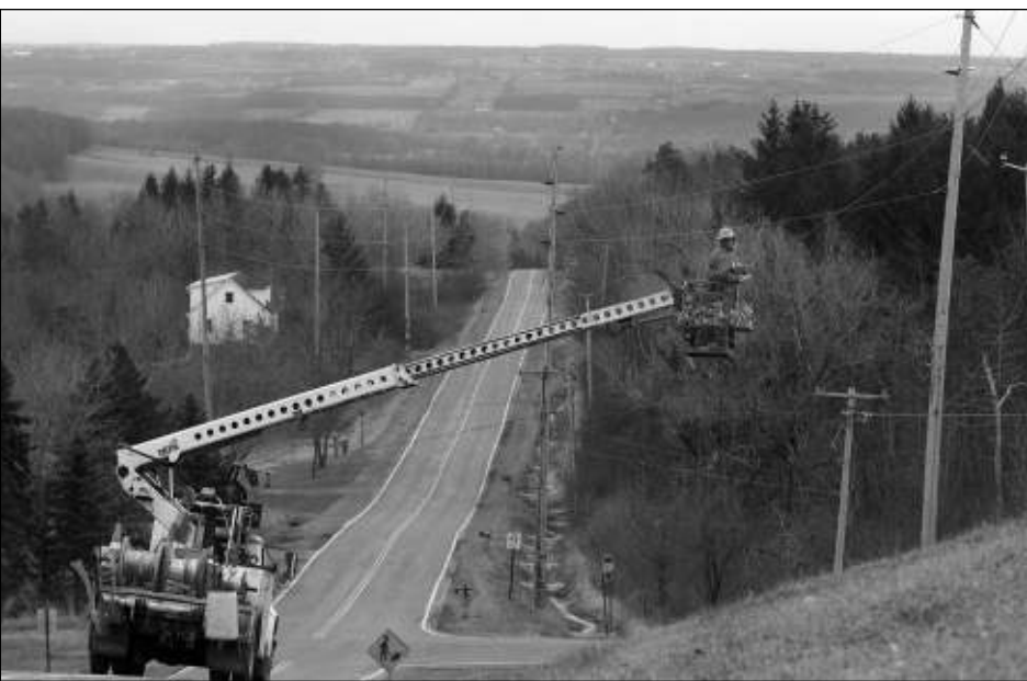
Daniel Bentley, of Rome, N.Y., runs fiber-optic cables along Goodale Road in Cheshire, N.Y.
