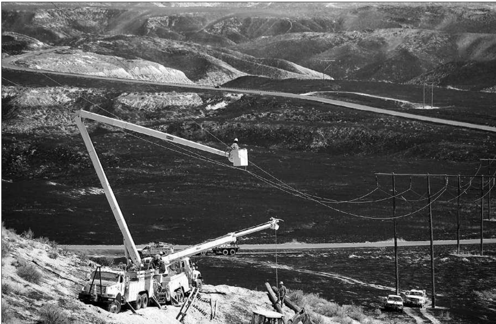
Idaho Power crews work on lines that run next to parts of the Oregon Trail at the Hagerman Fossil Beds National Monument on Wednesday. Many Idaho Power structures in the Hagerman area have been damaged by the Long Butte Fire.
