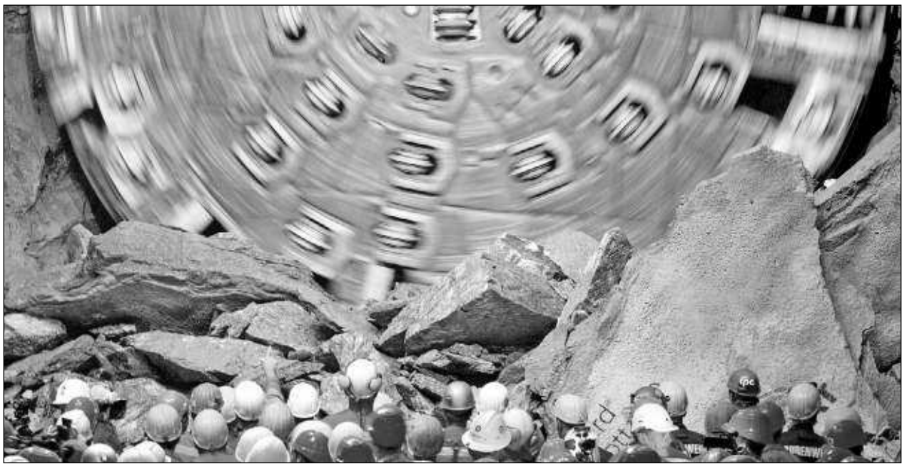
Miners watch the drill machine 'Sissi' after it broke through the rock, at the construction site of the NEAT Gotthard Base Tunnel on Friday. With a length of 35 miles crossing the Alps, the world's longest train tunnel should become operational at the end of 2017. AP photo
