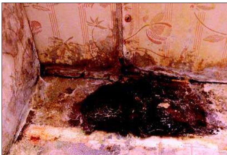
Mold under a vanity grew up to two inches high after a flood in Janice Bowman's bathroom.
