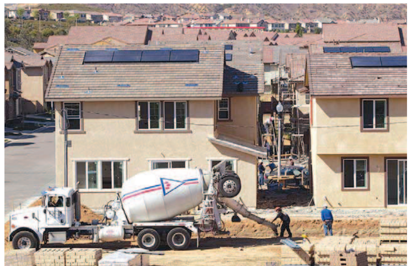
New homes are seen being built on March 15 at a development in Santa Clarita, Calif.
