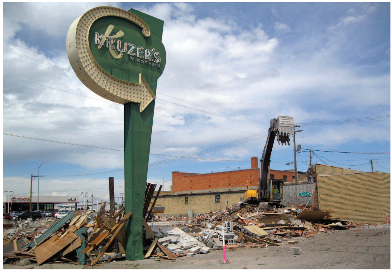
Workers with Boise-based AAI Demolition tear down the former Kruger's Nightlife location Wednesday along Shoshone Street in downtown Twin Falls.
