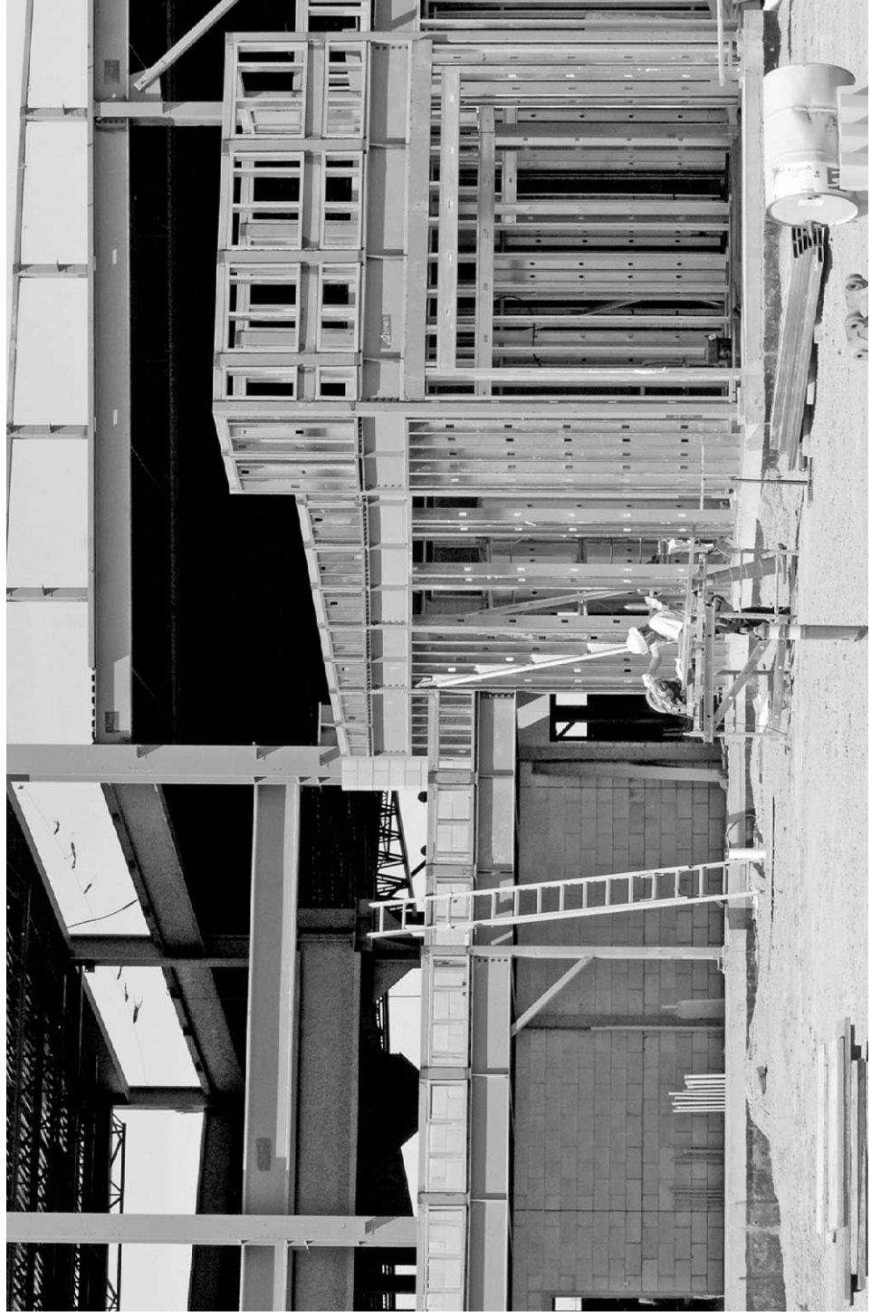
LAURIE WELCH • TIMES NEWS Construction was underway April 24 at the new Double L Manufacturing site west of Idaho Highway 27 in Heyburn. The facility is in the first urban renewal area established by the Heyburn Urban Renewal Agency.
