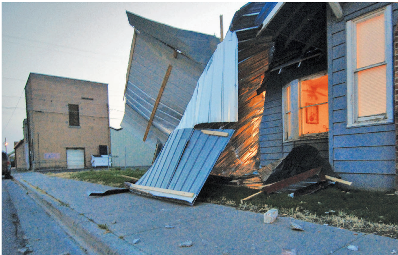
PHOTOS BY ED GLAZAR • FOR THE TIMES-NEWS (TOP) A large section of tin roofing hangs Monday night from the facade of Staci Vogt's home at 260 4th Ave E. in Twin Falls, after high winds tore it from an adjacent building. A cold front traveling across southern Idaho brought wind gusts as high as 51 mph, according to the National Weather Service. Sporadic power outages, small fires and fallen trees were reported across the Magic Valley.
