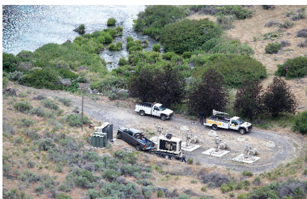
City crews use a generator to power water pumps at Blue Lakes on Tuesday.
