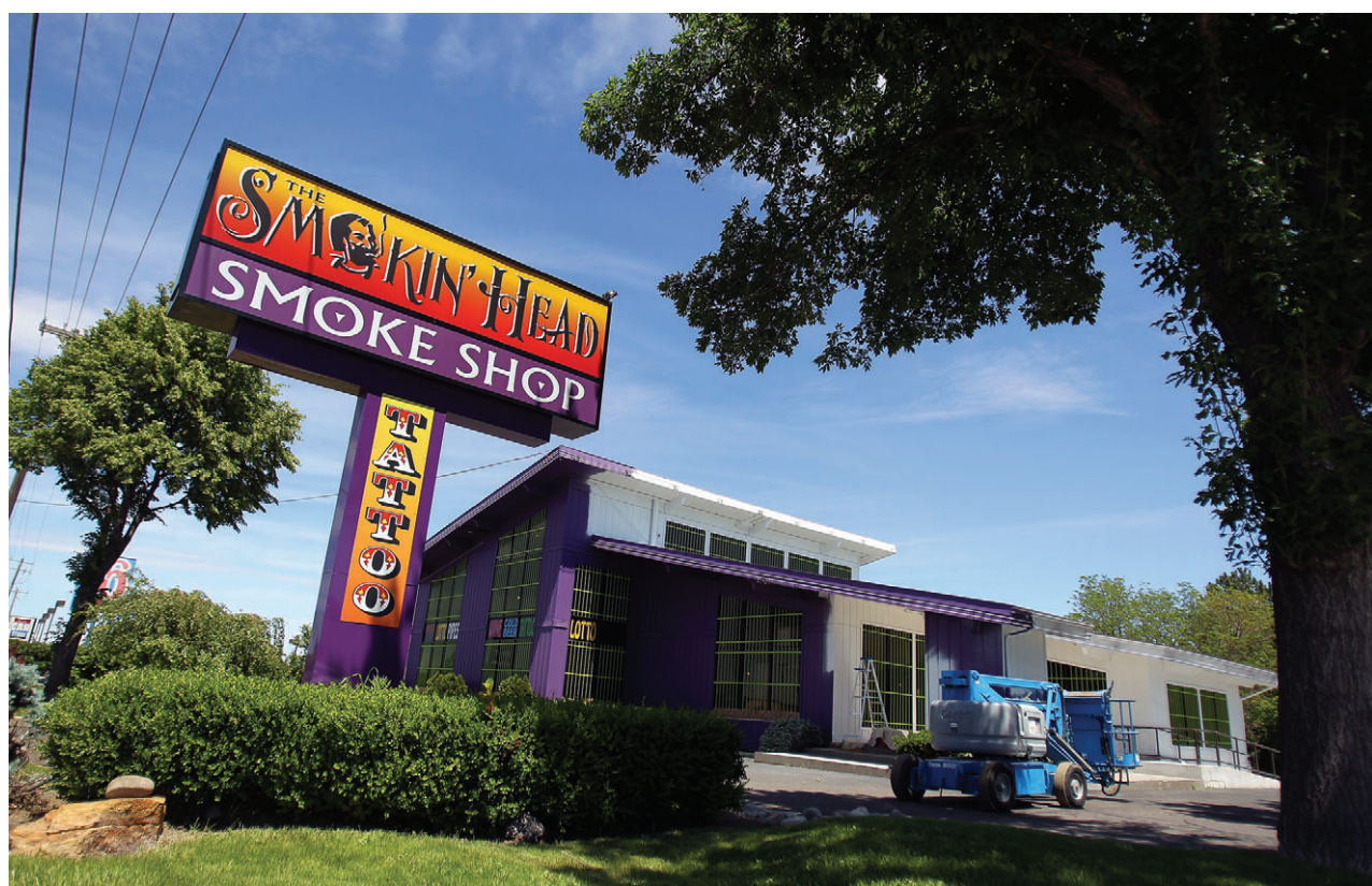
The Smokin' Head Smoke Shop gets a makeover while Fat Rat Tattoo moves into the building Thursday in Twin Falls.
