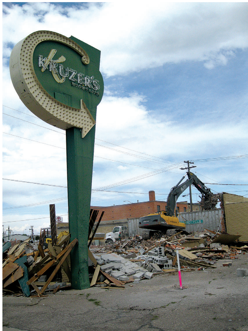
Workers with Boise-based AAI Demolition tear down the former Kruzer's Nightlife location in April along Shoshone Street in downtown Twin Falls.
