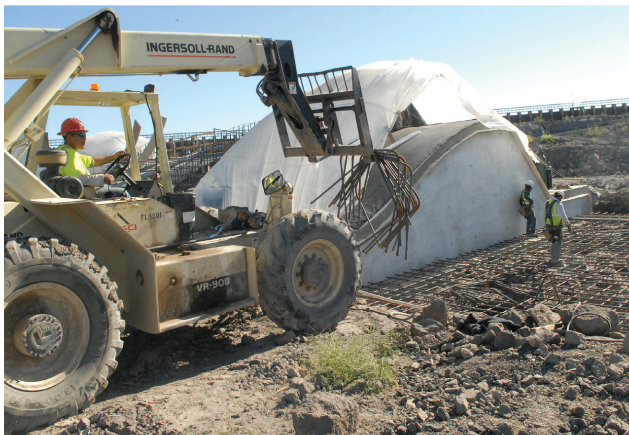
Workers install a rebar grid at the base of the south gated spillway at Minidoka Dam, part of an overhaul set to conclude in 2015. Care is taken to clean and prepare the foundation to prevent leakage under the spillway.
