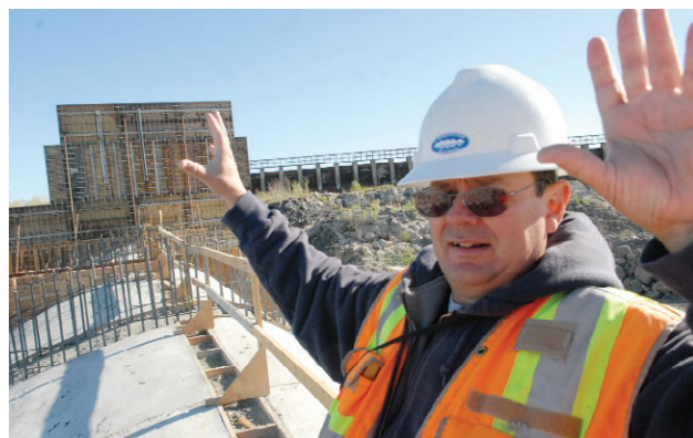
Bureau of Reclamation Resident Engineer Eduardo Lopez-Owsley explains the timeline Thursday for construction on the Minidoka Dam spillway project from the top of the new south gated spillway. This portion of the spillway will contain 12 gates and is the main water control structure for the dam.
