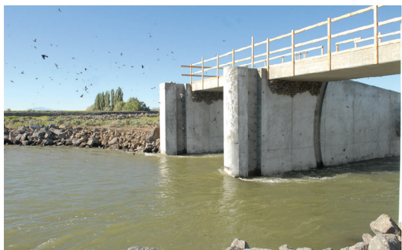
Dozens of swallows who are nesting on the new concrete structure of the Burley Irrigation District head works feed Thursday on mayflies.
