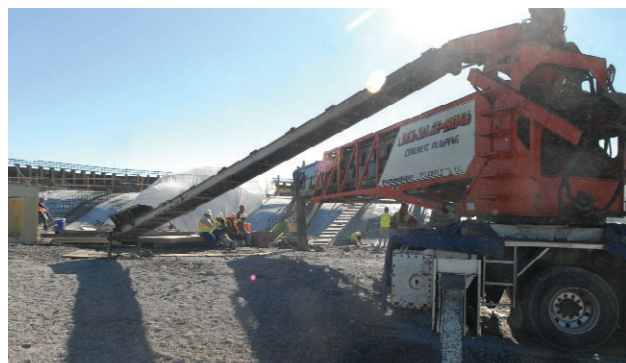
A Putzmeister Telebelt, one of two in the western United States with a conveyor belt designed to telescope out 130 feet, is used to place concrete Thursday.
