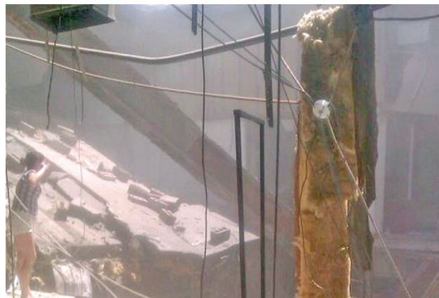
ASSOCIATED PRESS A woman checks out the damage after a roof collapsed at the Algo Centre Mall in Elliot Lake, Ontario, Saturday.
