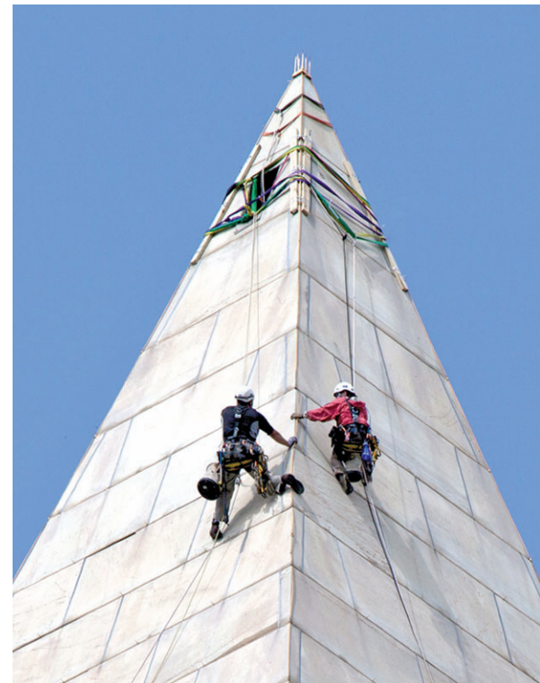
MICHAEL E. RUANE, NATIONAL PARK SERVICE - THE WASHINGTON POST Inspectors examine the Washington Monument in Washington, D.C. in September 2011, to access damage caused by an earthquake on Aug. 23, 2011.
