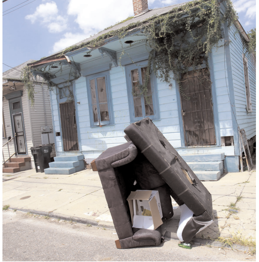
ASSOCIATED PRESS A blighted home, which is managed by the Louisiana Land Trust, is seen on Dumaine St. in New Orleans.
