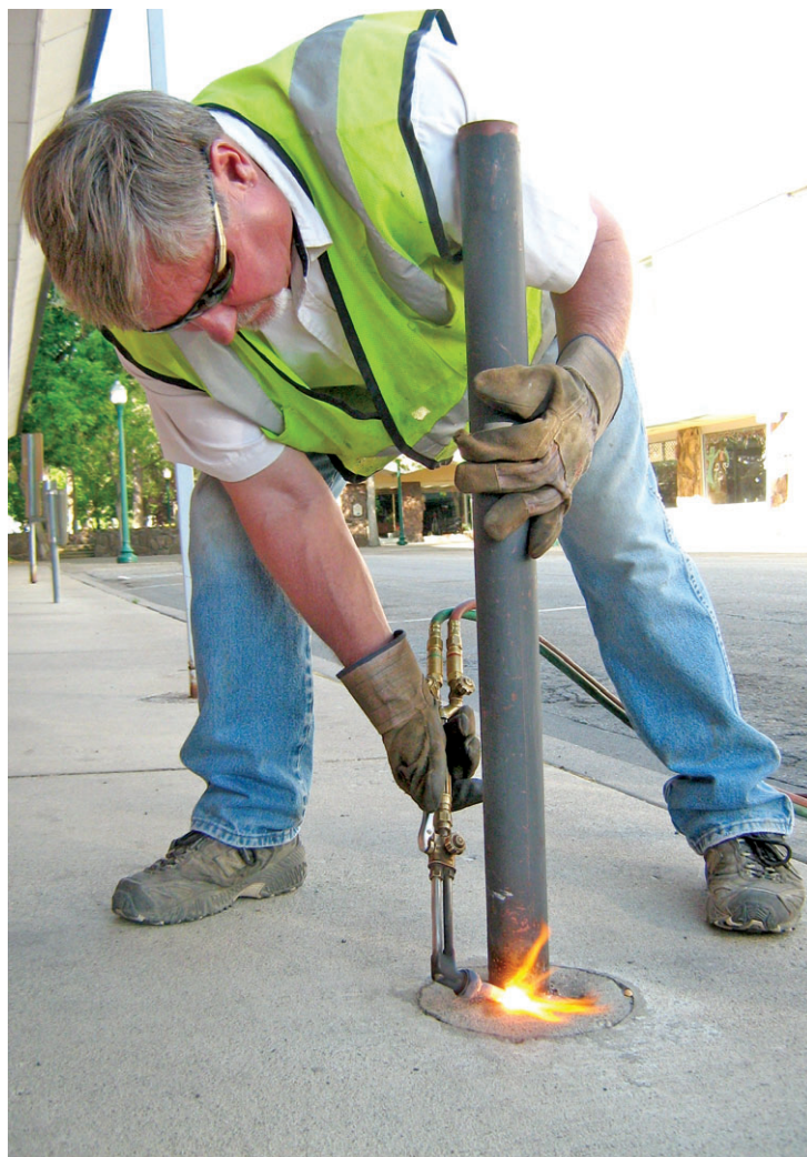
LeRoy Hartgrave, lead worker for the Twin Falls City Streets Department, removes a parking meter post from a downtown street July 1. With the city's long-debated downtown parking meters removed, discussion has turned to how to address the area's parking needs without them.
