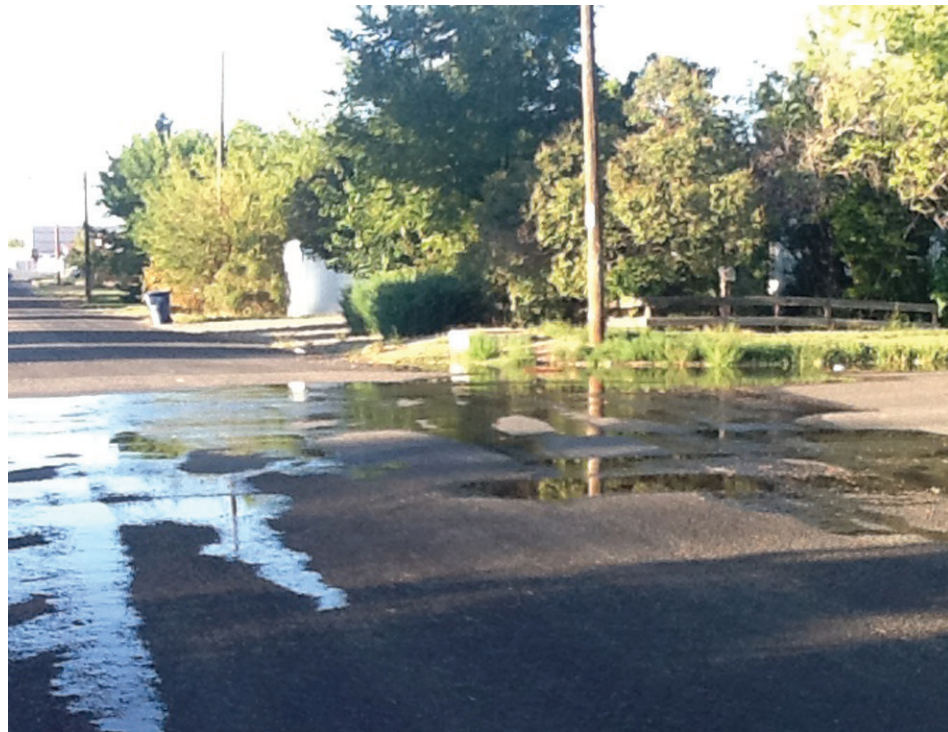
Water spilled from a broken water main is seen Monday evening at the corner of South Cedar Street and West Avenue F in Jerome, one block down from where crews repaired the damage.
