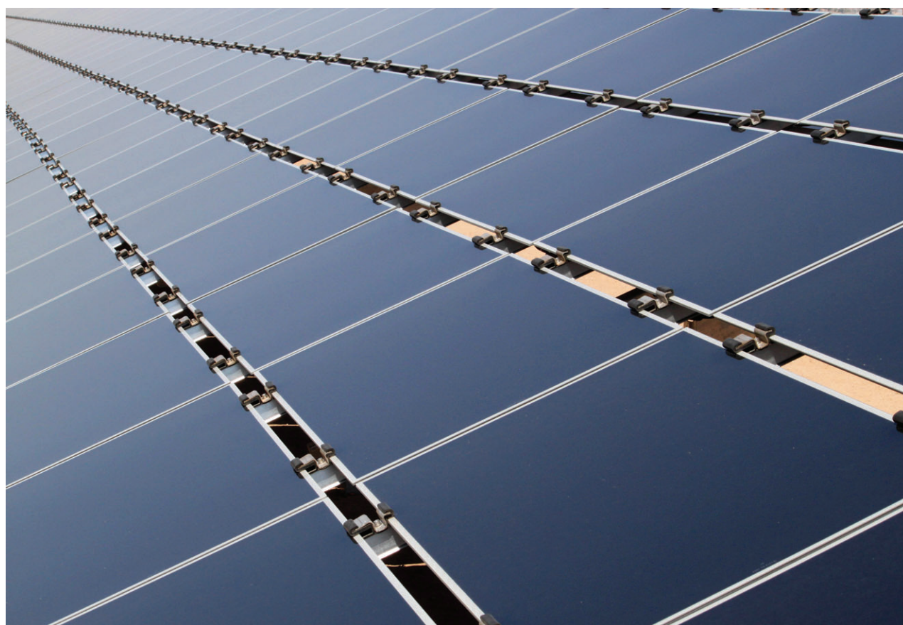
Solar panels are seen in Albuquerque, N.M.
