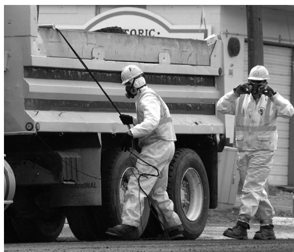
Road workers wear protective gear against possible asbestos contamination as they load material from a road resurfacing project in downtown Libby, Mont.
