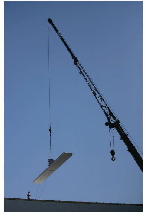
A construction worker helps guide a crane Friday at High Desert Milk in Burley.
