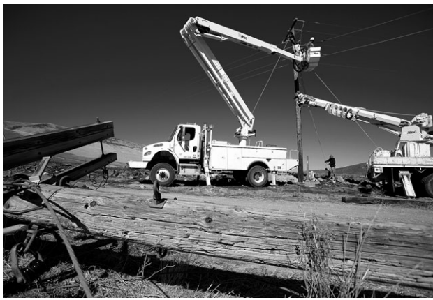
A Raft River Electric crew replaces a power pole Thursday damaged during an August wildfire near Elba.
