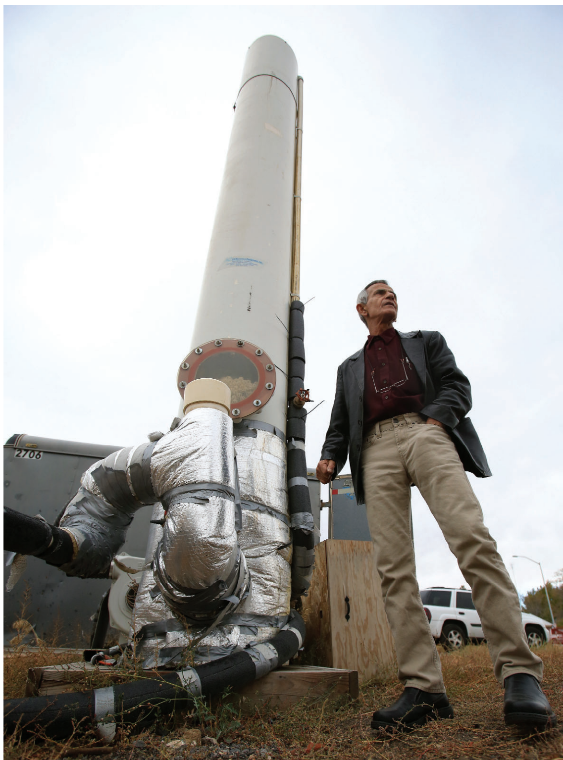
Saiid Dabestani, owner of Enviro-Mont in Twin Falls, stands next to a system that cleans up gas that has leaked into the ground at a former gas station along Washington Street North.
