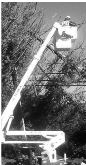
Idaho Power is a part of the Western Mutual Assistance Group. Before Hurricane Sandy made landfall, the Long Island Power Authority reached out to the group.
