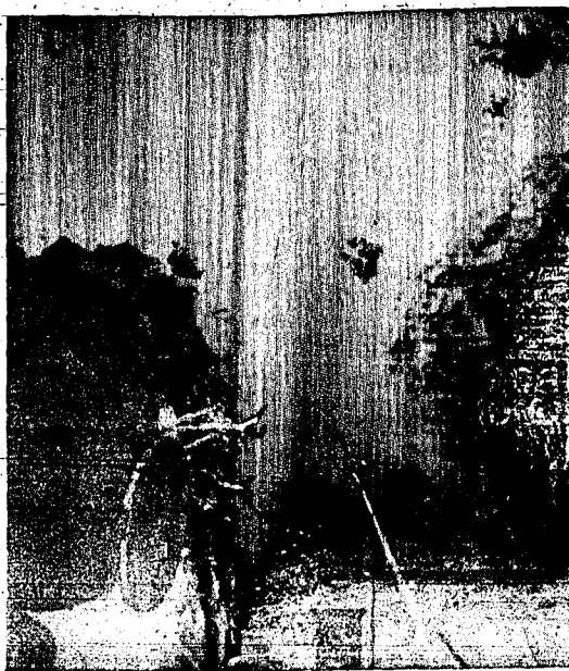
Workers labor at the end of the trench installing pipe at the north end of Blue Lakes boulevard north. There are crews installing pipe at several locations in Twin Falls. Work on the new Twin Falls sewage disposal plant and the new sewer system will be completed in about 18 months. The plant is located in the Snake river canyon, north of Twin Falls. (Staff photo-etching)
