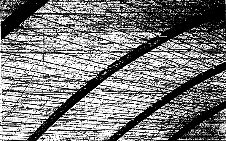
STEEL BEAMS OF the huge covered stadium being constructed at Idaho State University, Pocatello, make an interesting pattern for the Times-News camera. When completed the structure will permit thousands of spectators to view football and basketball games regardless of the weather conditions. It will be the first structure of its kind in Idaho. Initial football game in the new stadium is slated for late November.
